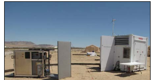
Micro-grid with battery storage
